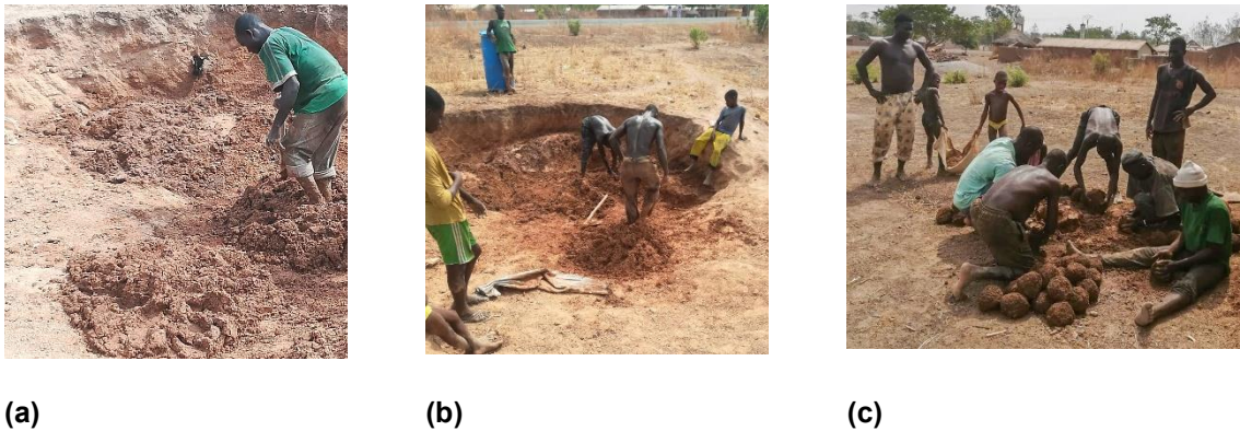
Figure 11: Pictures Showing the Excavated Earth Being Mixed After Watering And The Clods Of Earth Being Formed For Construction
