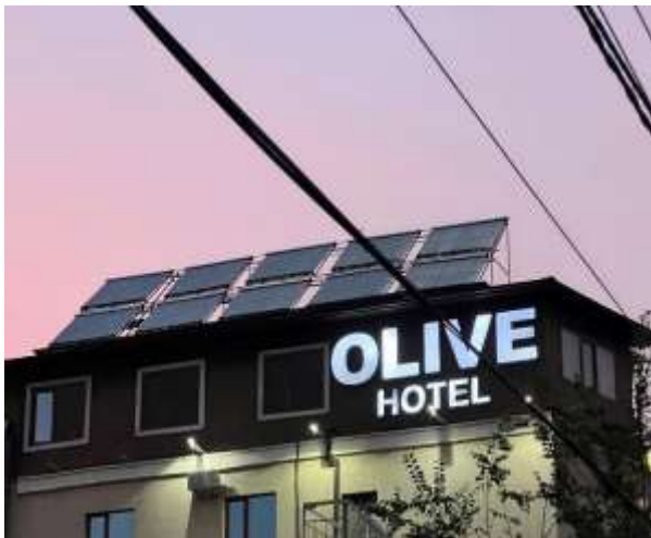
Figure 11. Solar collectors on the roof of the Olive Hotel
