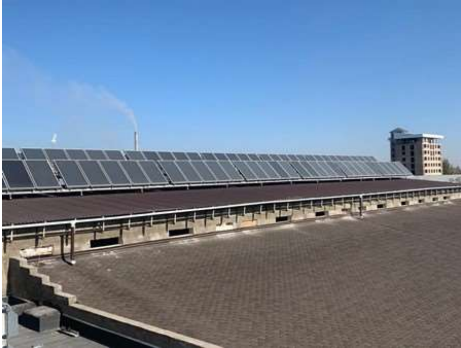
Figure 12. Solar collectors on the roof of the Dasmia Fitness Family fitness centre
