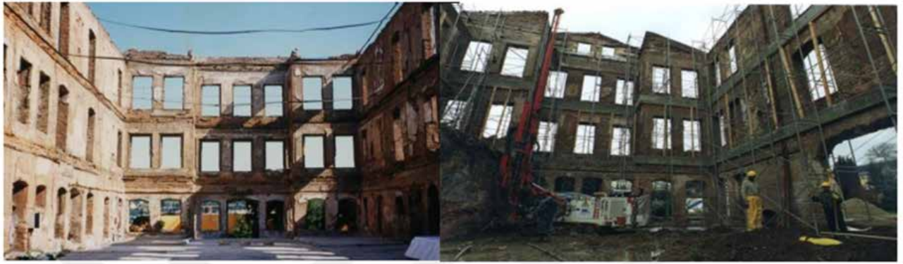
Figure 5: The Historical Esma Sultan Mansion After the Fire.
